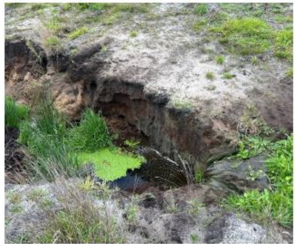
Photo 3-7 Erosion present along drainage line
