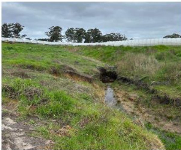
Photo 3-6 Drainage line in eastern paddock revegetation area
