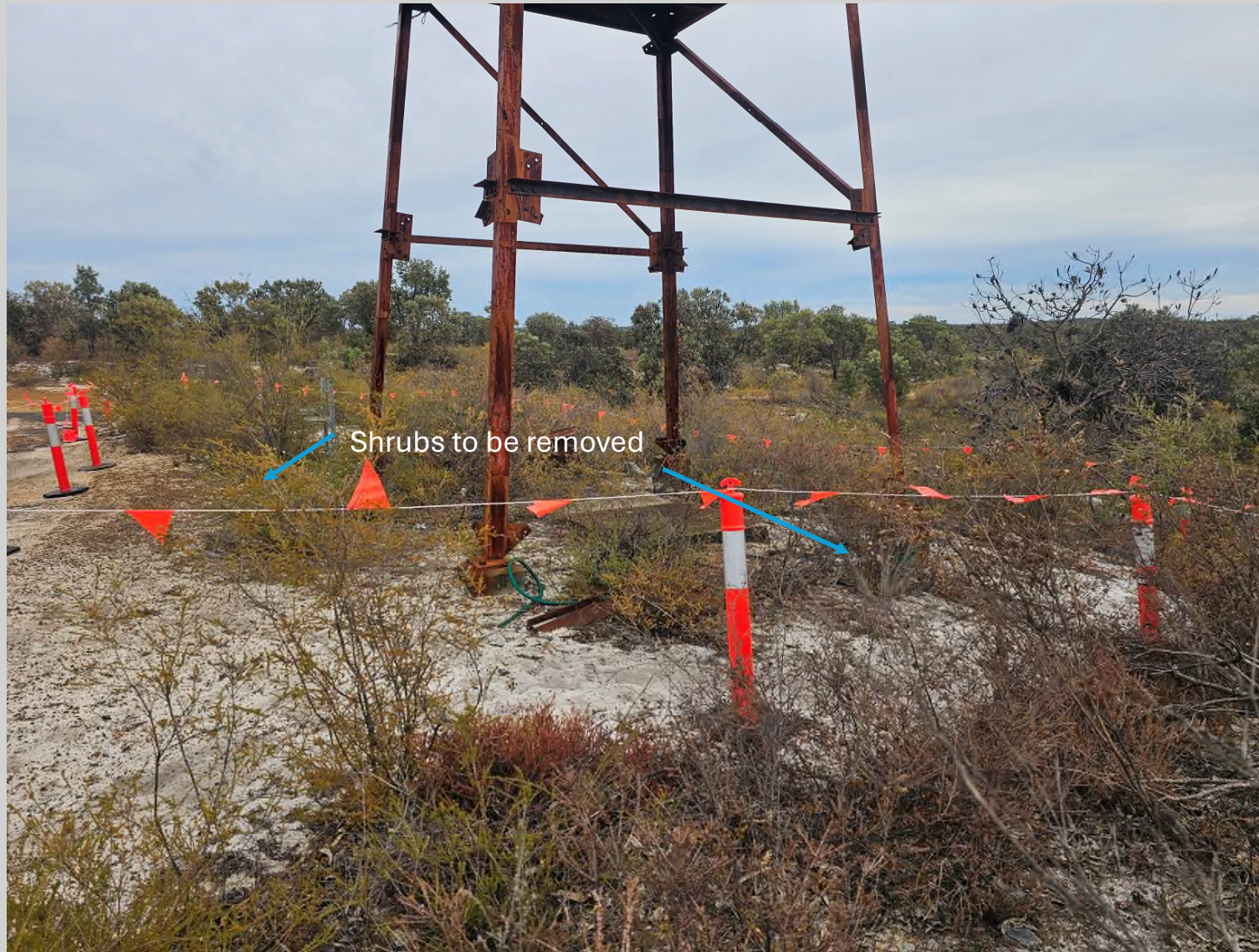
Photo 12 – ACM Impacted Area 1C Looking South East Towards Tower
