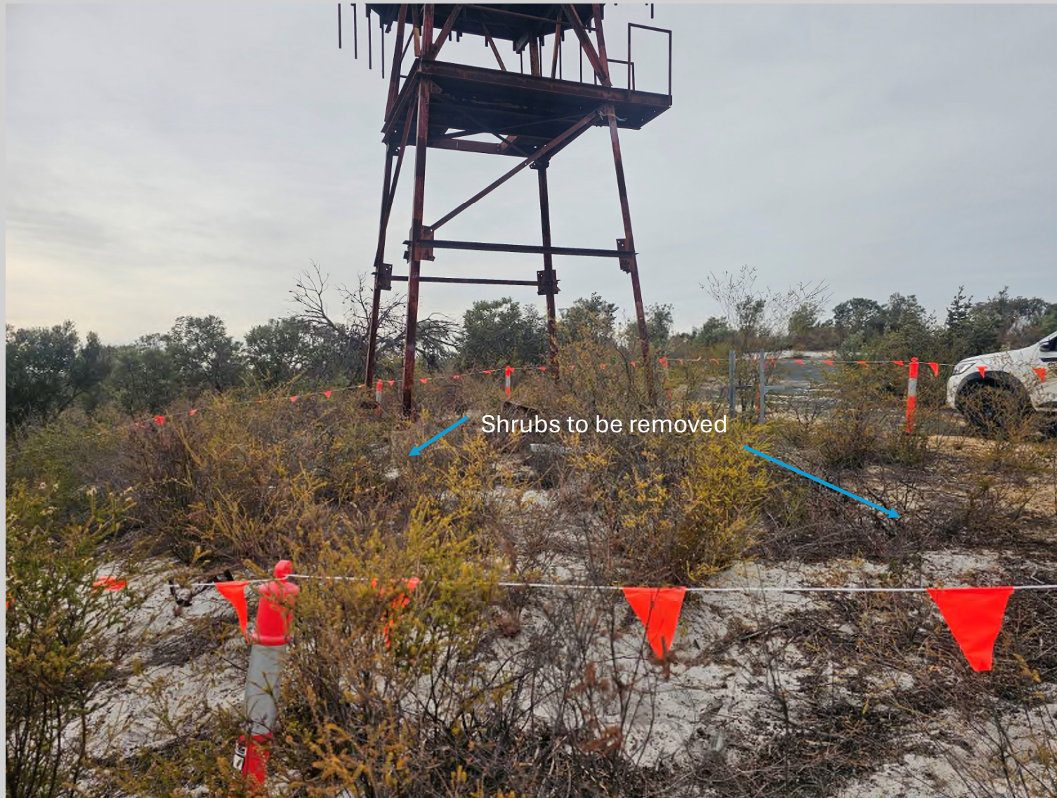
Photo 11 – ACM Impacted Area 1C Looking South East Towards Tower
