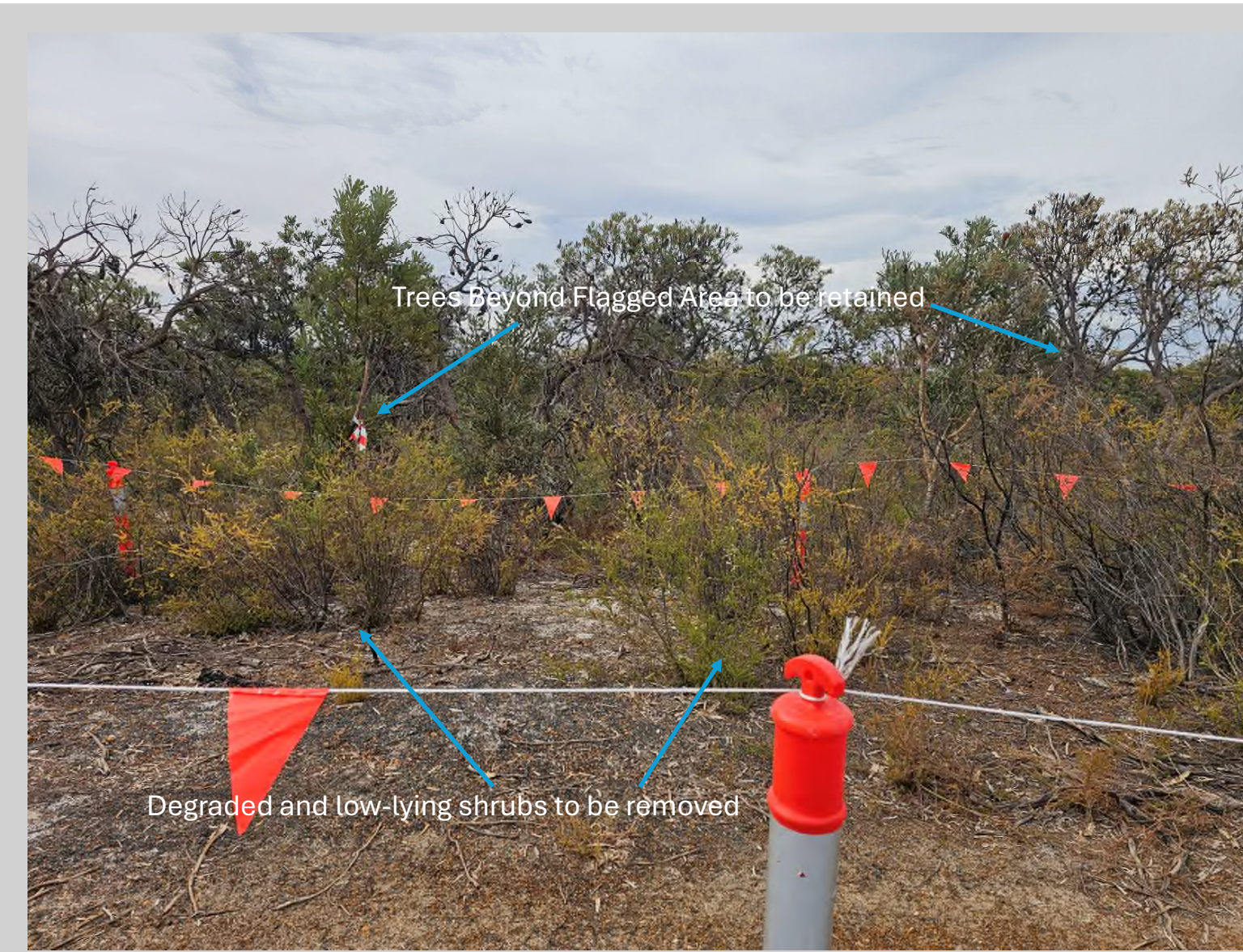
Photo 8 – ACM Impacted Area 4B
