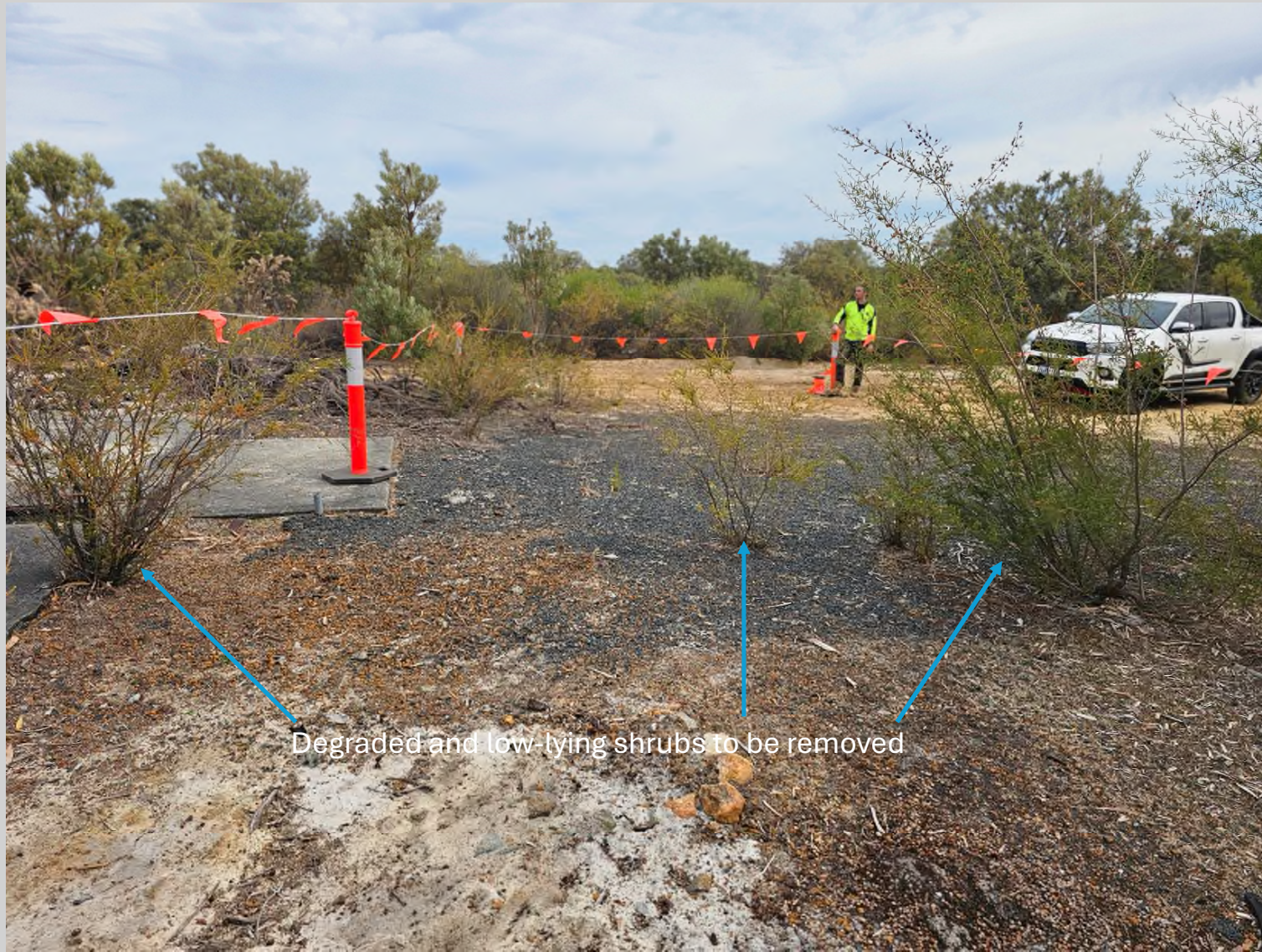
Photo 9 – ACM Impacted Area 3
