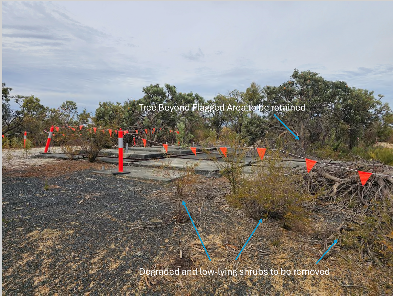
Photo 10 – ACM Impacted Area 3
