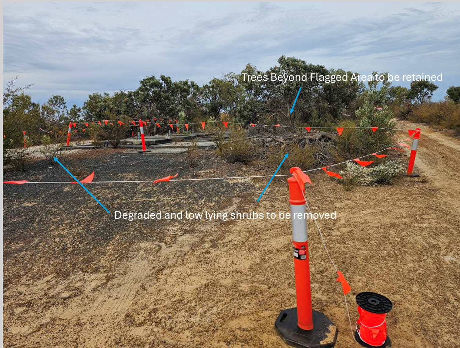
Photo 1 – ACM Impacted Area 3
