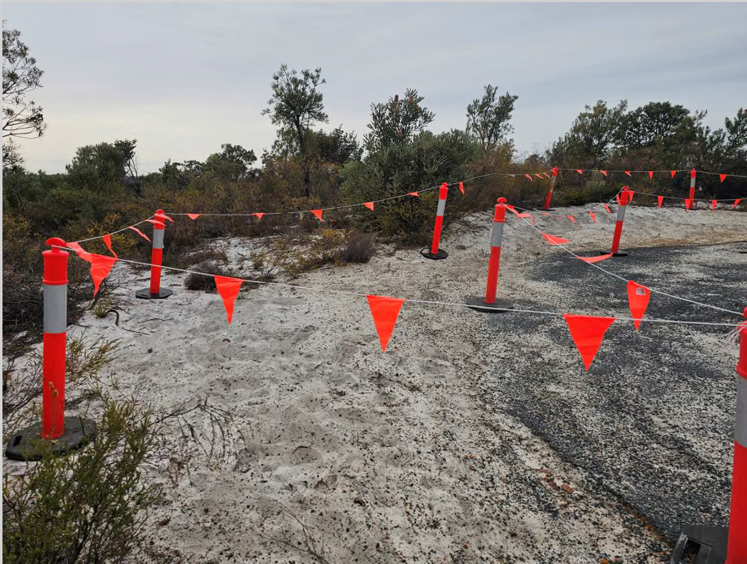
Photo 17 – ACM Impacted Area 1D Looking South
