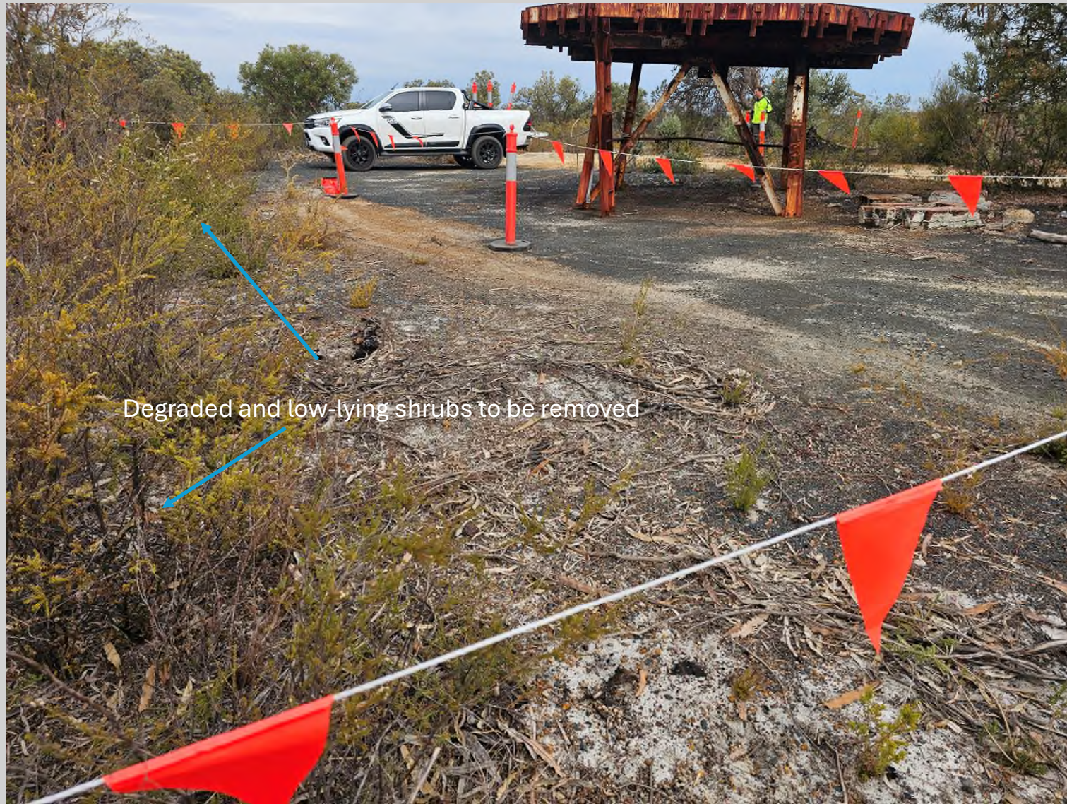
Photo 13 – ACM Impacted Area 4B
