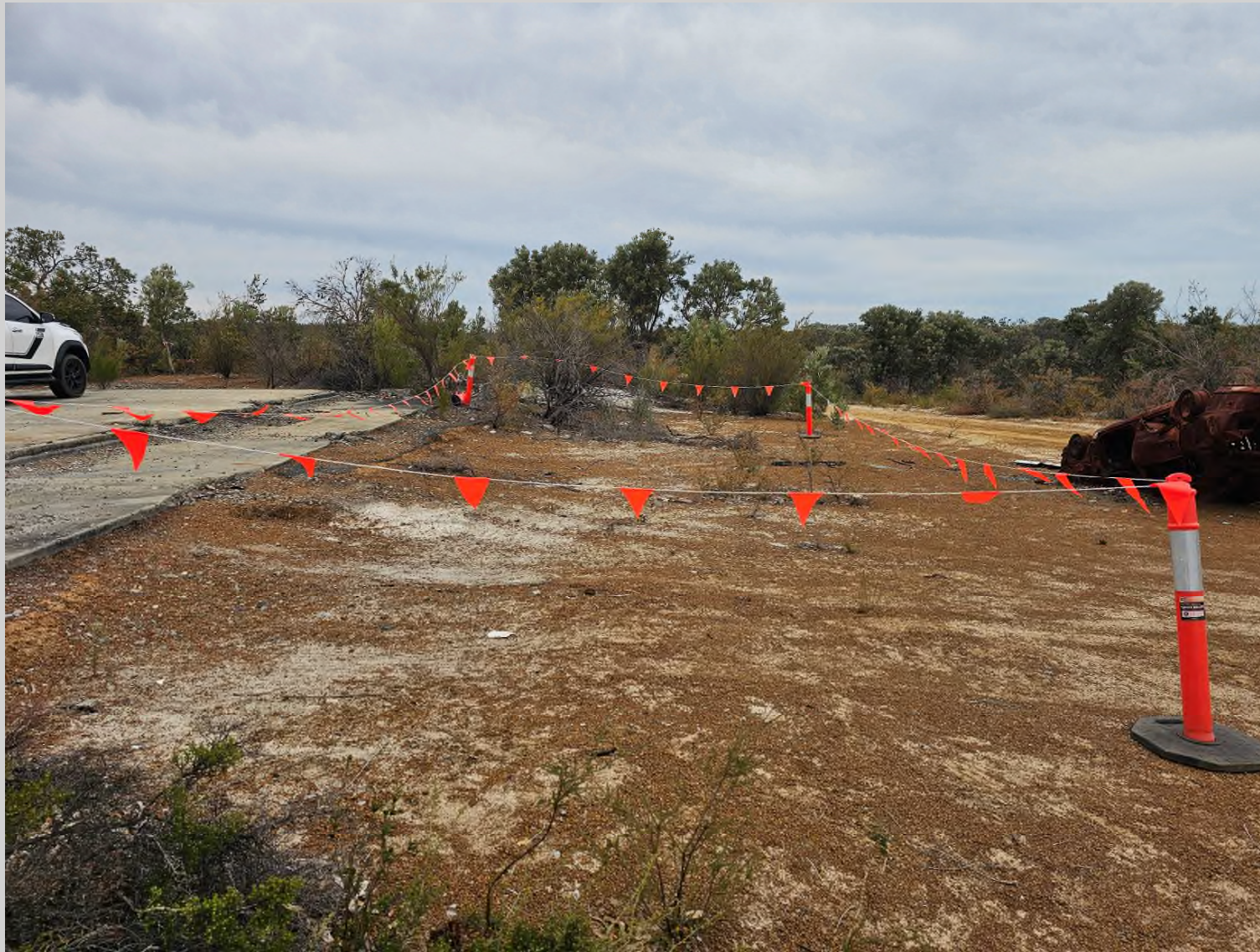
Photo 30 – ACM Impacted Area 1G Looking South
