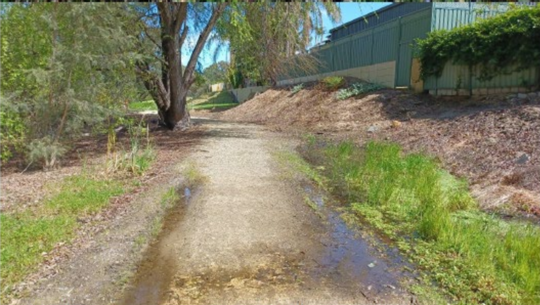
Current incidences of Typha growing within 3 m of the fire track, residential properties to the north of the fire track
