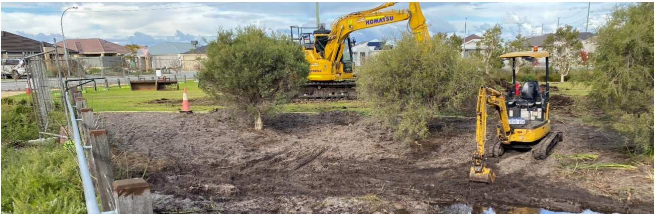
Figure 5: Vegetation removal within the drainage swale at Sheaf Park for the City of Armadale as part of the Newhaven Stage 1 project (2021).
