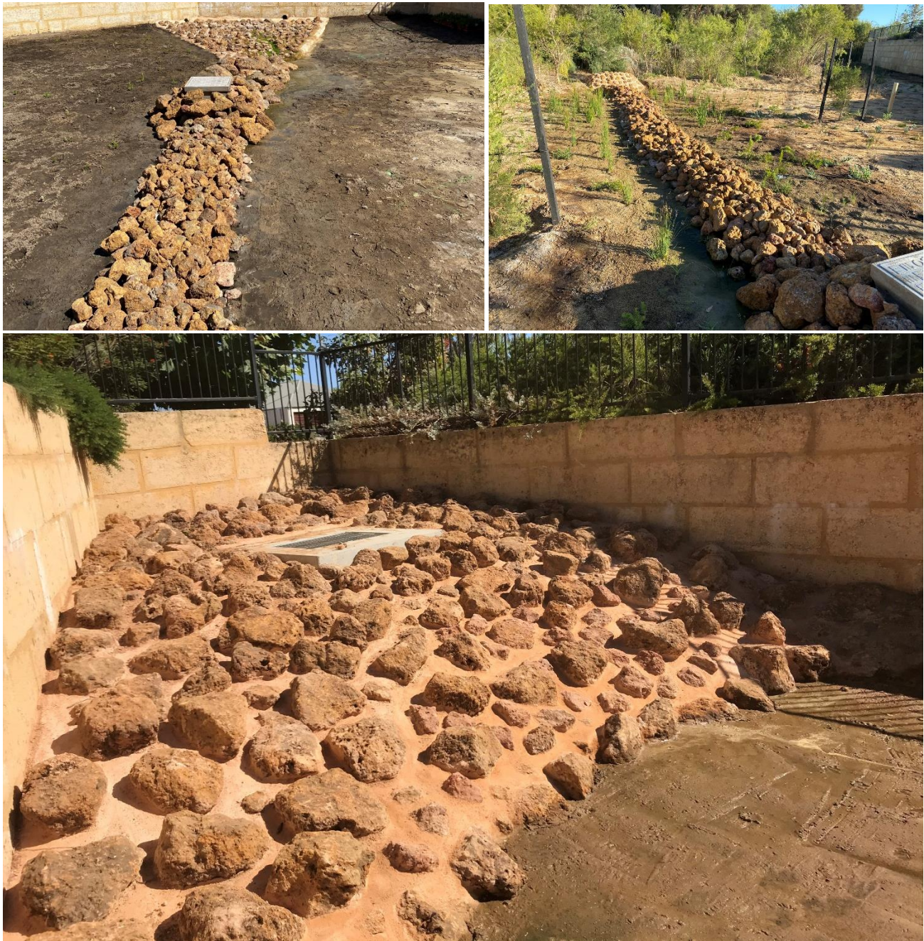
Figure 7: Installation of laterite rockwork and mortaring at McPhail Park for the City of Armadale as part of the Newhaven Stage 1 upgrade works.
