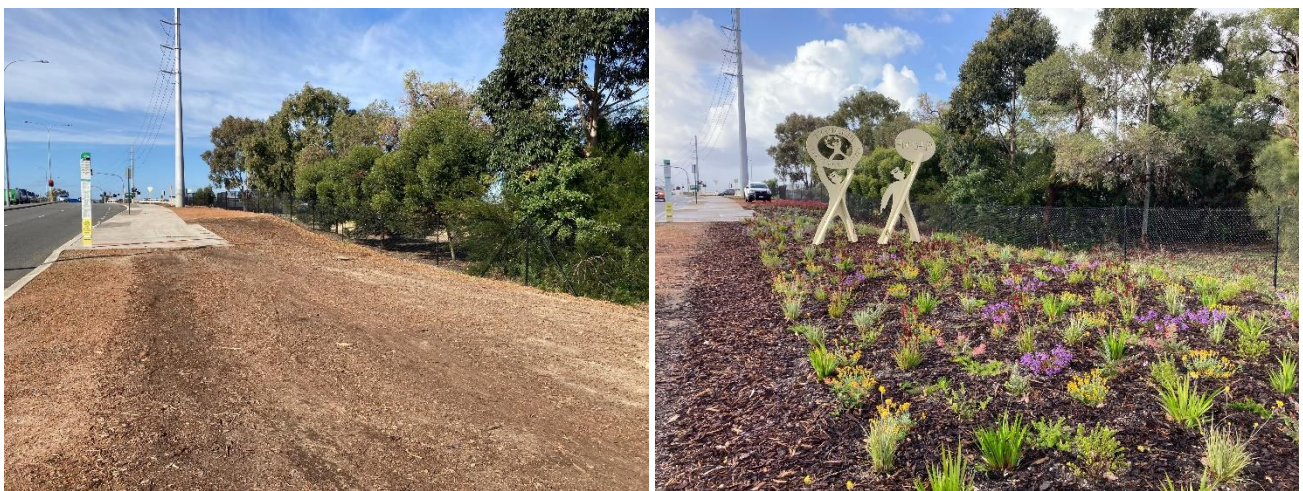
Figure 15: Before ( left ) and after ( right ) mulching and landscaping works at the Abernethy Road Entry Statement for the City of Belmont.
