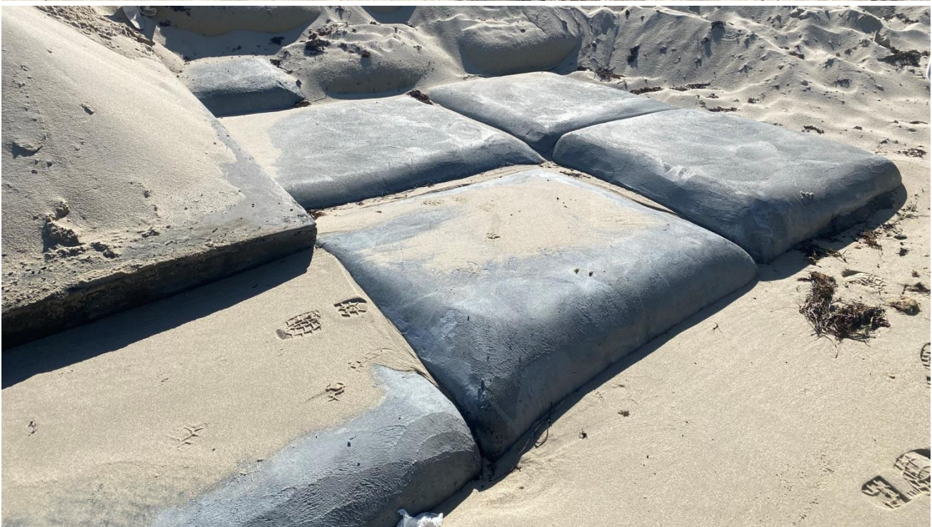
Figure 12: Concreting works undertaken by Total Concrete at Mettam’s Pool; forming concrete by hand to tie into the existing GSC revetment (2021).
