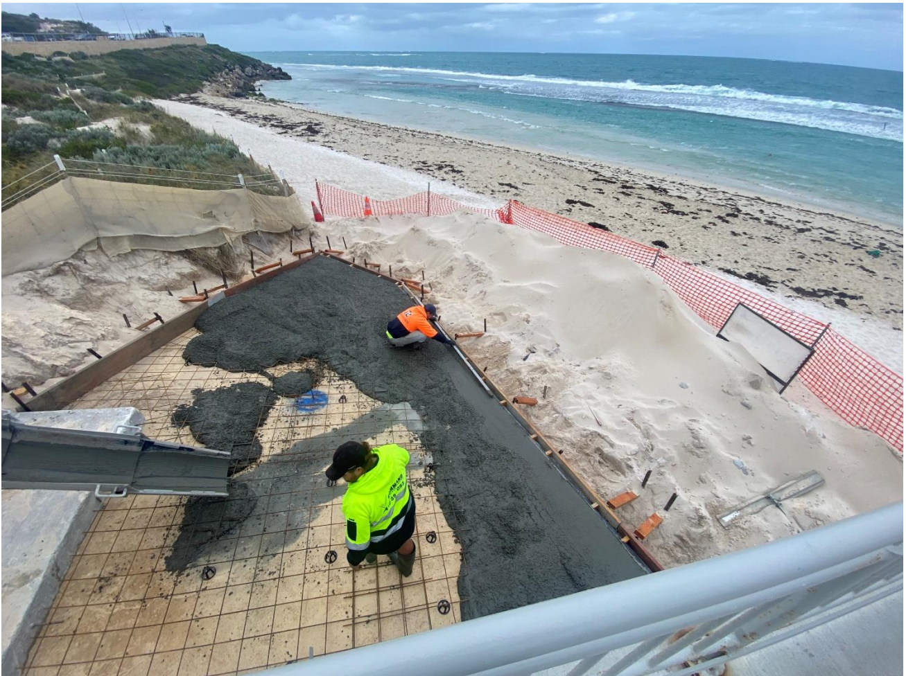
Figure 11: Concreting extension to the vehicle access way at Yanchep surf lifesaving club undertaken by Total Concrete as part of Natural Area’s Stair remediation project (2023).
