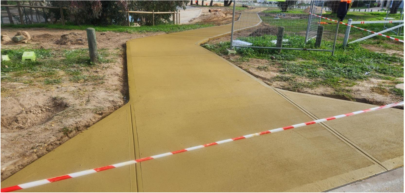
Figure 10: Total Concrete was sub-contracted to install a Boral Maze footpath to the City of Kalamunda’s specifications at Natural areas project site in Wattle Grove (2023).
