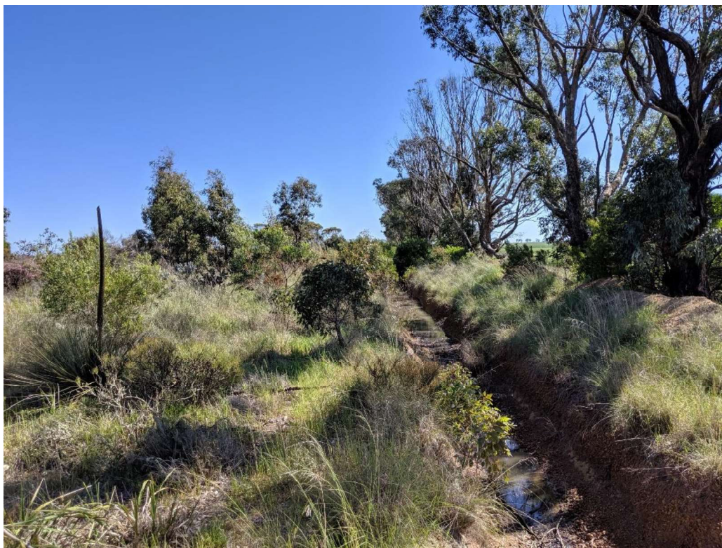
Figure 13. Photo of degraded area along the edge of the road reserve, with recently dug drainage line present.
