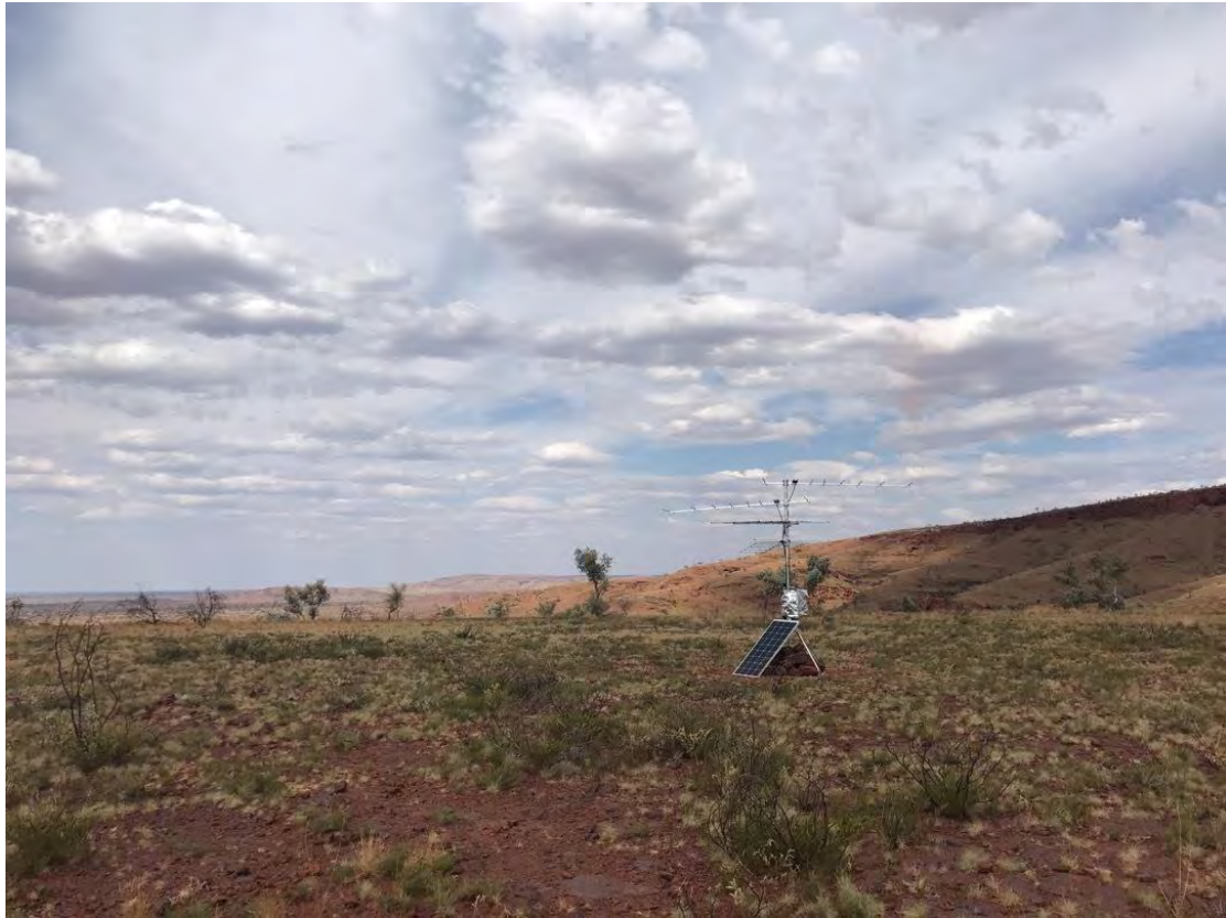
Plate 3.1 VHF receiver tower installed in the Study Area
