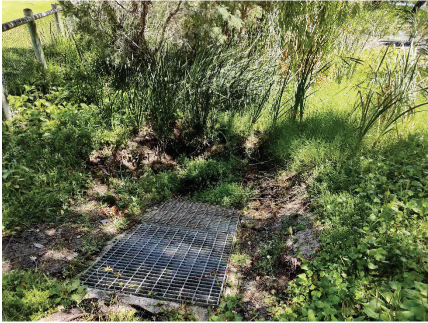
Plate 21: Wolinski Park in Mullaloo, Typha growth proximal to drain. Potential for future overgrowth to impact infrastructure and hydrology. Taken from Eastern fence line.
