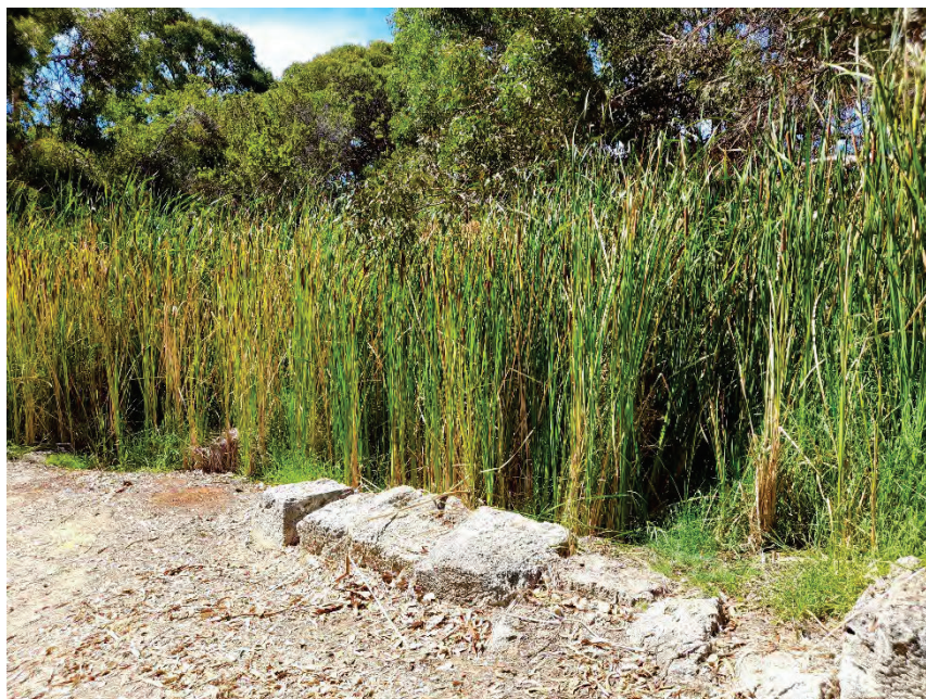
Plate 2: Blue Lake Park in Joondalup, Stream overgrown by Typha, causing damage to the structure and watercourse. Taken from Southern side of stream.
