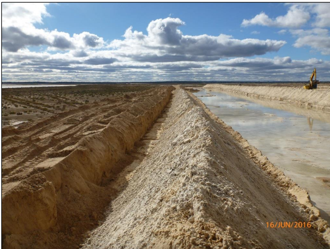
Plate 14: Strip mining sequence showing of quarry excavation (RHS), gypsum windrow (middle) and topsoil material as outer windrow (LHS)
