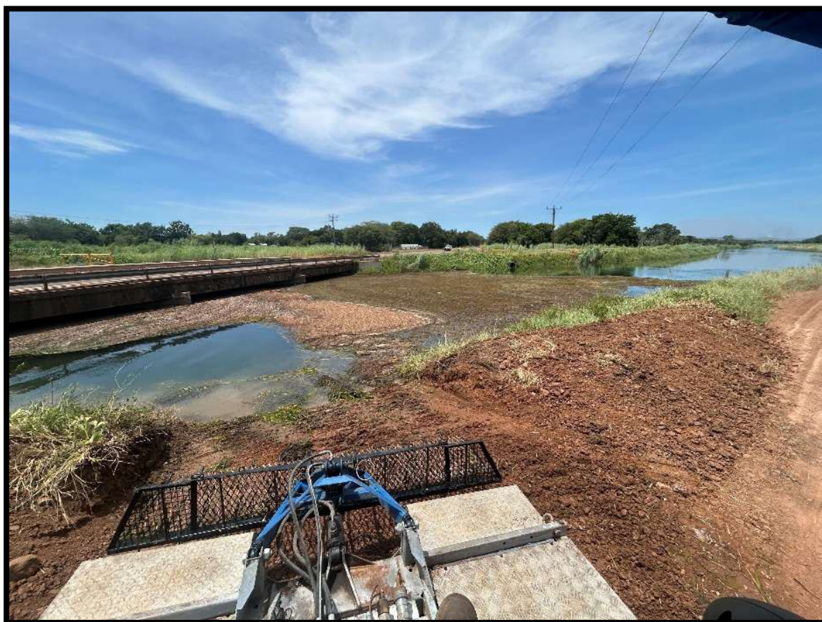
Figure 5: Before the clearing of weeds in channel - the waterway channel has minimal flow, weeds impeding flow and the commencement of eutrophication to the channel. The Truxor operator has clear visuals to identify any fauna or flora species within the direct clearing channel (Hydroscape Environmental, 2025).
