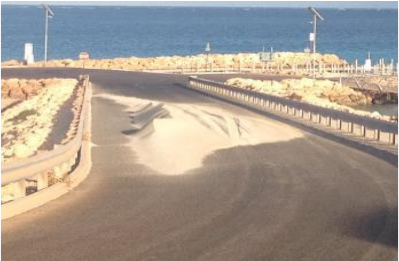
Figure 1.2 Build-up of seasonal sand deposition on the Coral Bay Boating Facility causeway road
