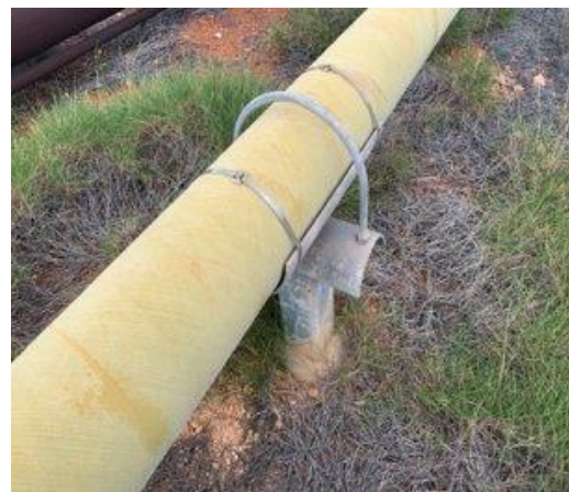
Photograph 3-12: Pipeline (>100 mm) pipe supports with buried foundations
