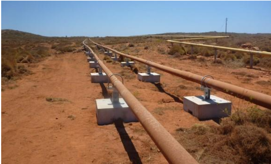
Photograph 3-3: Pipelines (>100 mm) and pipe supports
