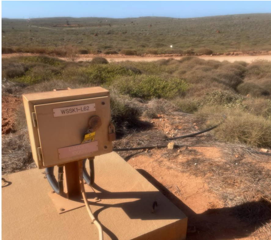
Photograph 3-6: On-ground power cables exiting well lease
