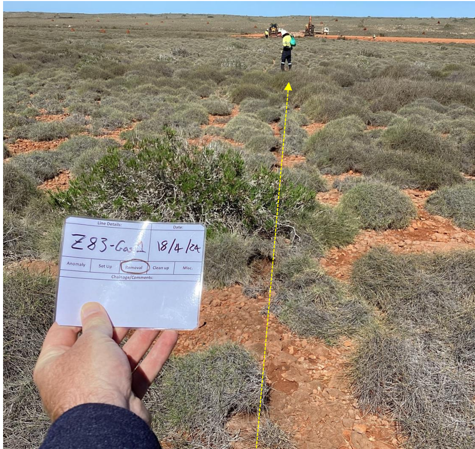
Photograph 3-9: Post flowline removal (pulled) ground disturbance (yellow line shows position of removed flowline)
