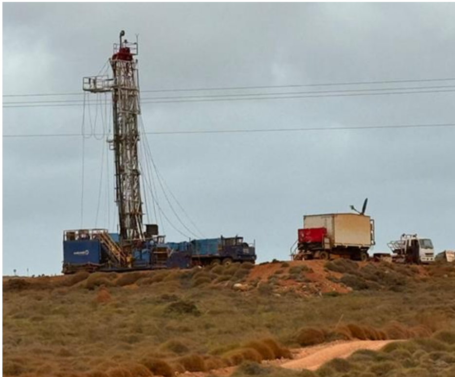
Figure 3-1: Example of a mobile rig used for workovers and plug and abandonment activities
