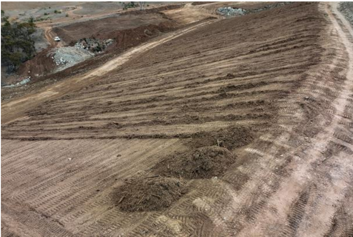
Figure 4. Rehabilitation site preparation utilising local native mulch (Galaxy Resources Pty Ltd, 2024a)
