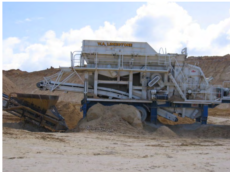
Typical mobile plant location on the floor of the excavation with near vertical faces
