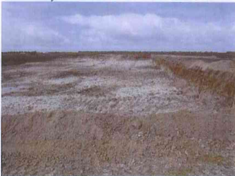
Shallow topsoil and loam over pallid zone clays in main detention basin
