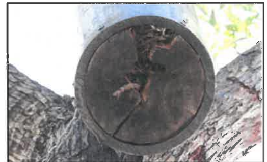
Artificial hollow base needing repair. Photo by Christine Groom
