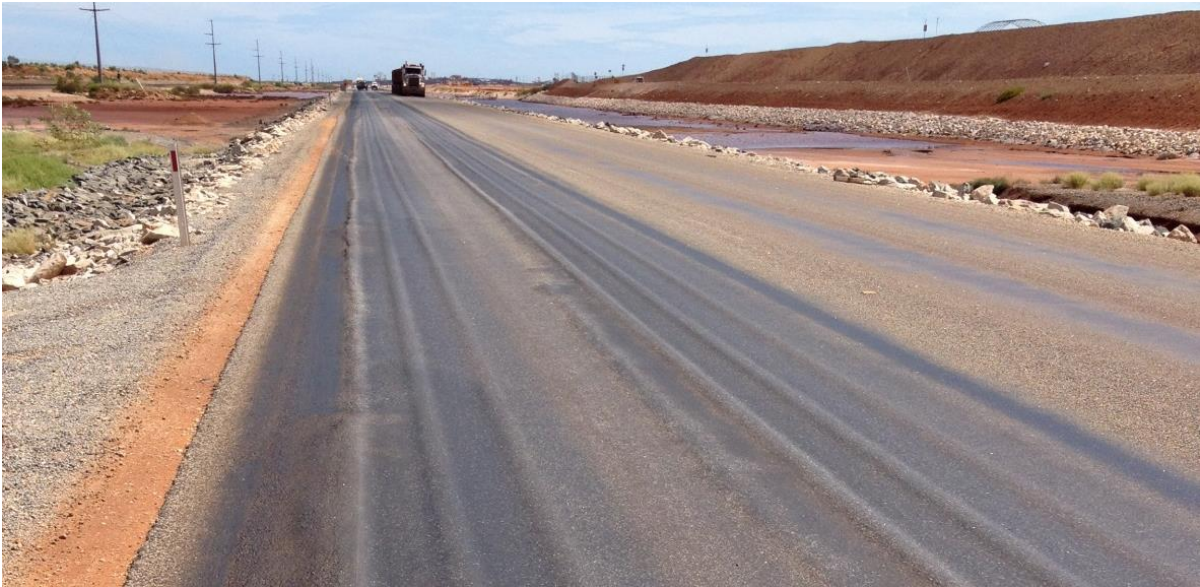
Figure 1: Typical pavement rutting on Utah Road.
