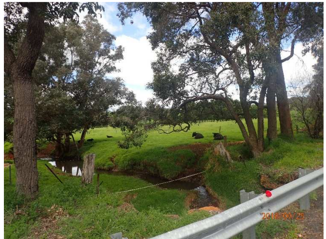
Figure 3 – Culvert crossing showing the watercourse within the application area showing lack of riparian vegetation
