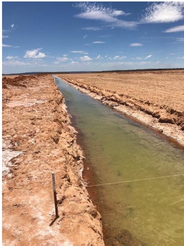
Figure 4: Example of trench infiltration (picture taken from Beyondie SOP Project)
