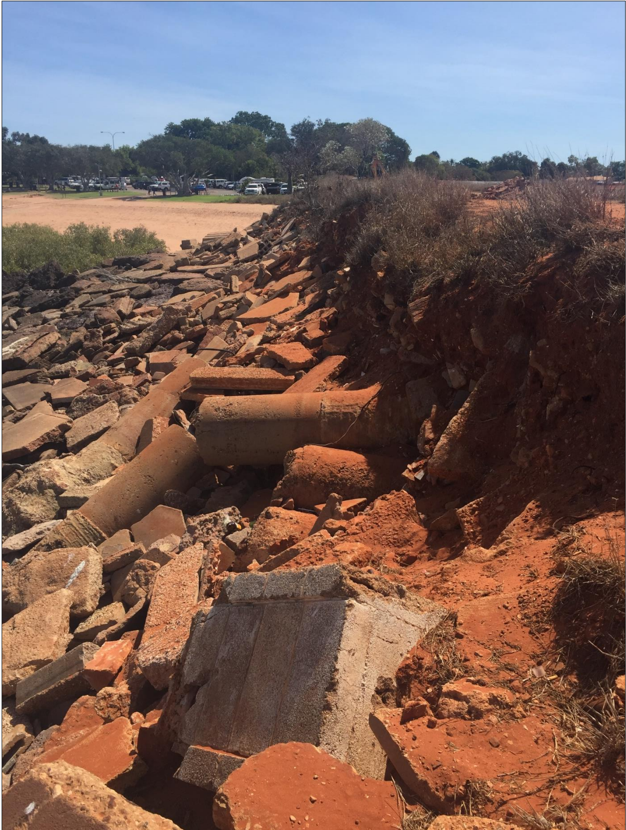
Plate 2: Evidence of erosion at Seaward end of Town Beach Jetty (MBS Environmental 2019)
