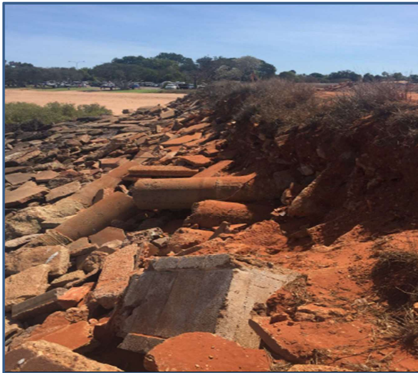
Figure 2 Photo from south side of Groin, facing Northwest, shows sparse vegetation and lack of soil profile (MBS environmental, 2019).
