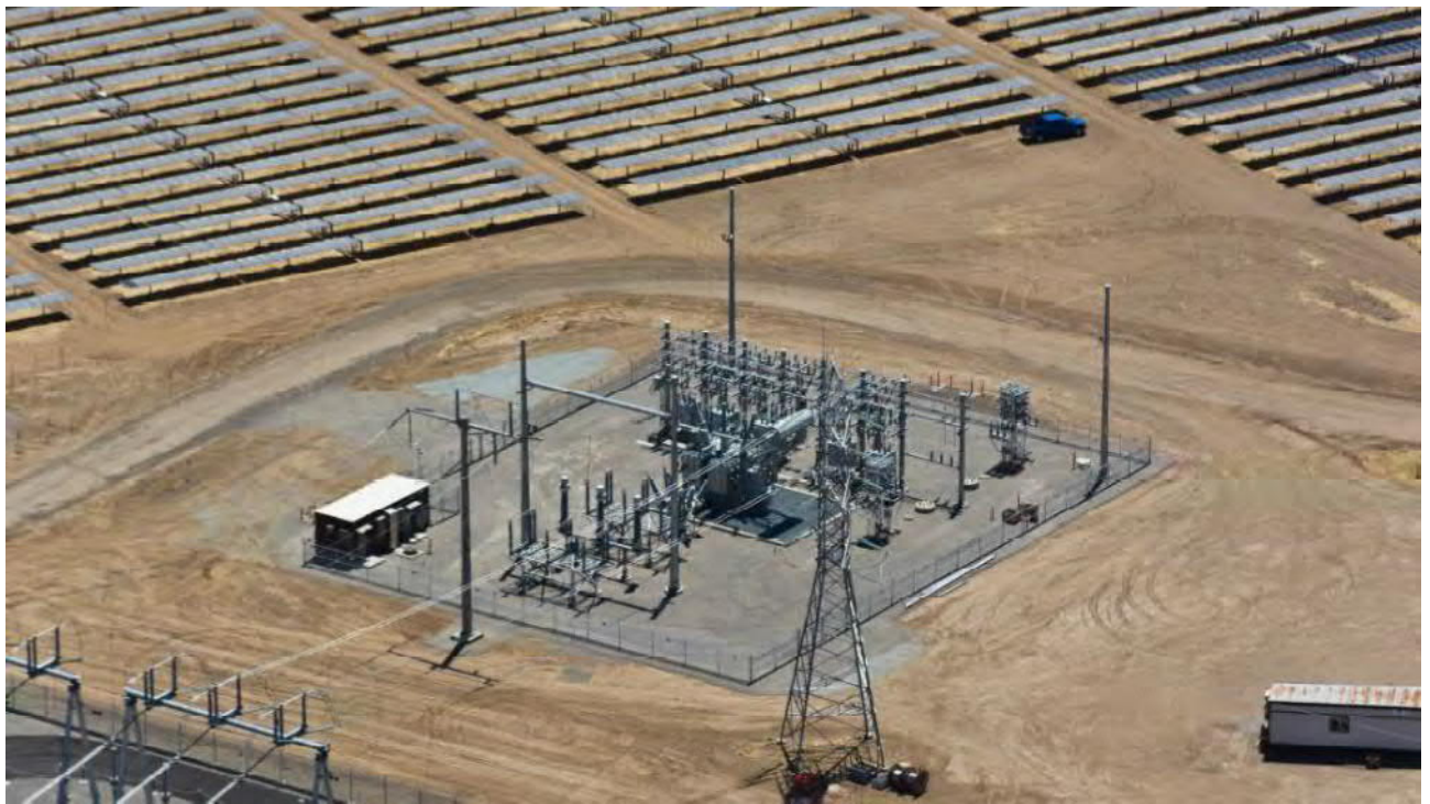
Figure 10 Typical example of a Solar Farm Substation.
