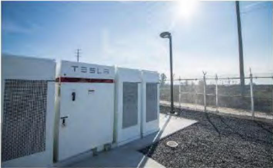
Plate 6 Typical battery storage
