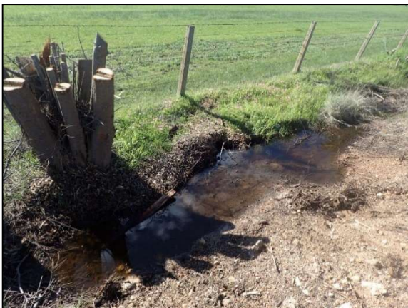
Photo 7: standing water within the application area
