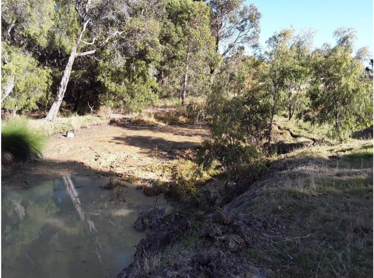
Figure 1 Slumping and erosion of the eastern bank. Significant cracks have developed causing the side to collapse.
