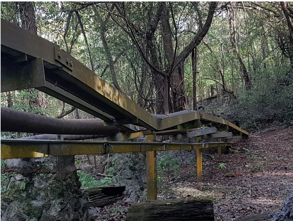
Figure 2 Damage to the pipeline due to recent tree fall over the pipeline
