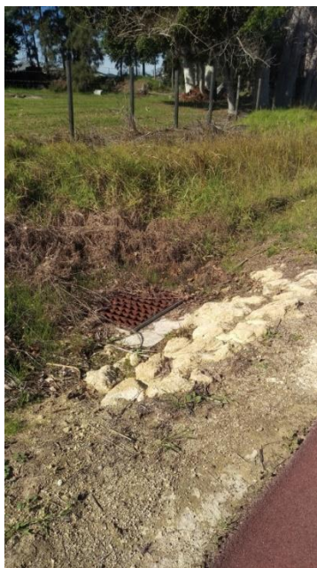
Plate 1: Open drain with limestone located outside of Lot 35 (within 20m 'offset' buffer area).
