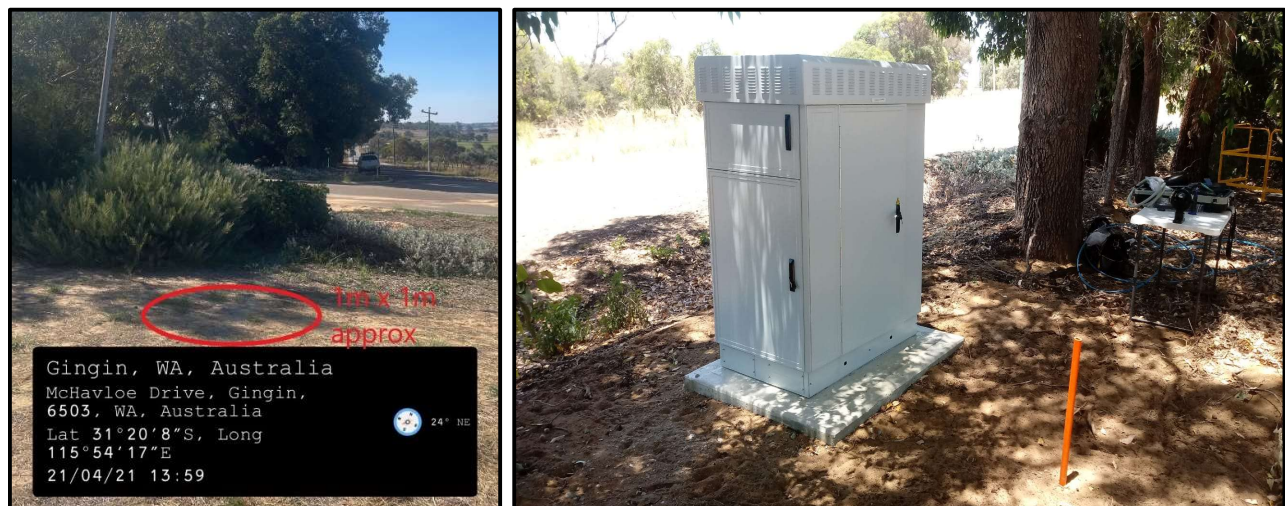
Figure 2 - The proposed directional drill pad location within the application area, located south of McHavloe Drive (left). The location of where the sub-surface directional drill will terminate at the orange conduit adjacent to the existing telecommunications cabinet (right) (Opticomm Pty Ltd, 2021b)
