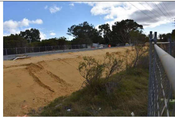
Photo 9: Completely Degraded vegetation –Skeet Road
