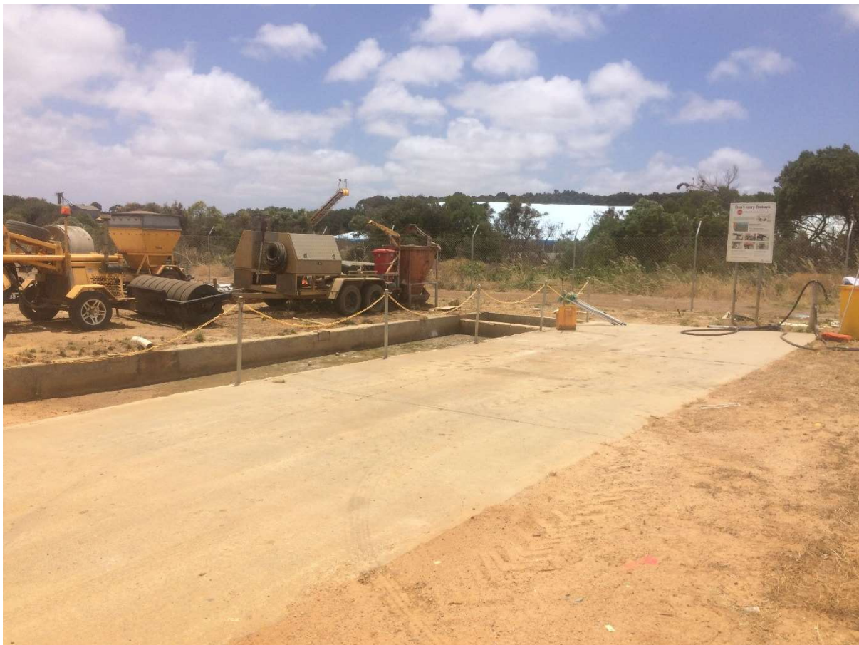
Figure 1: Shire of Esperance Depot vehicle washdown bay
