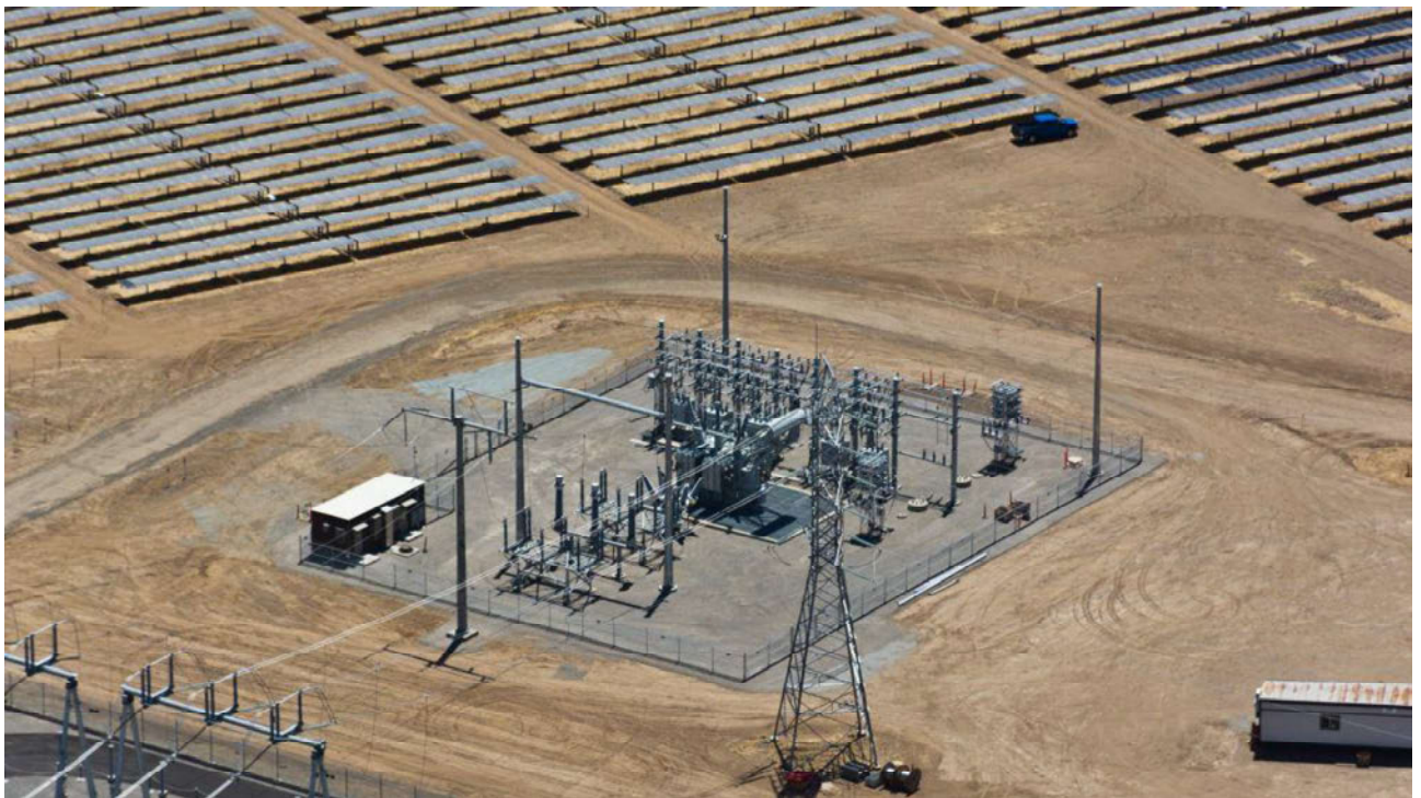
Figure 10 Typical example of a Solar Farm Substation.
