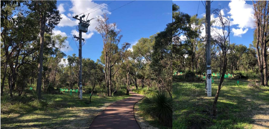
Figure 9 - These photos show the existing pole and transformer (S177236) that will be replaced. There is one small dead tree (2m) located close to the power pole. This photo also shows the location of the revegetation area to the east behind the power-pole.
