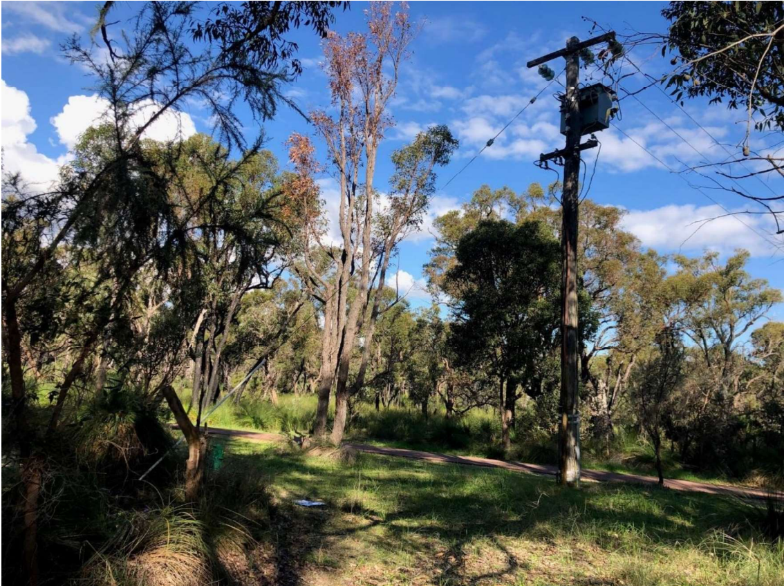
Figure 10 – View south of the existing pole and transformer (S177236) that will be replaced.
