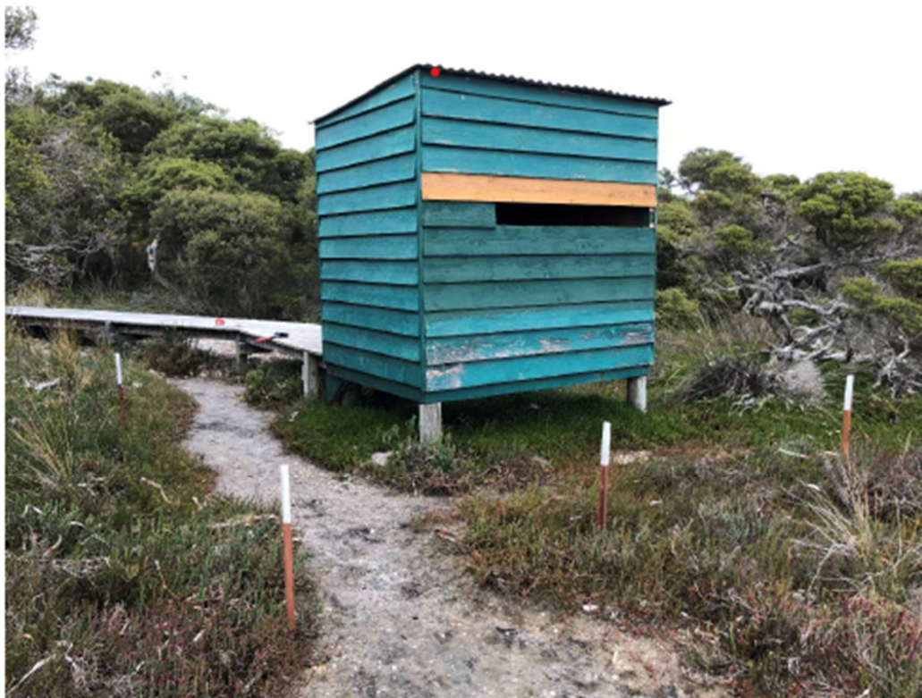
White pegs indicate approx. platform area – 12 holes to be dug for posts. No other clearing. Please note the vegetation that is still growing underneath the existing structure.
