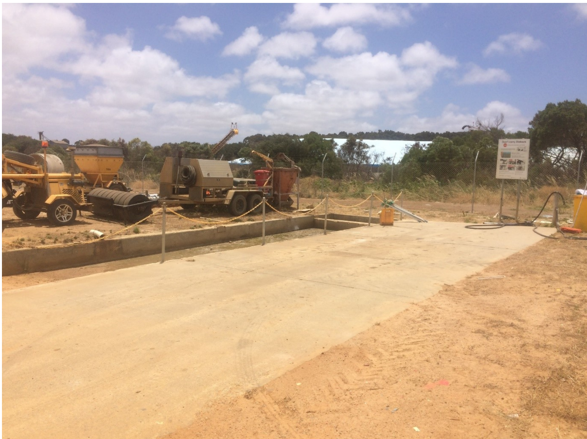
Figure 1. Shire of Esperance Depot vehicle washdown bay
