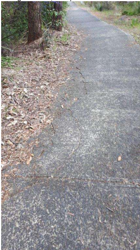
Figure 14. Photographs of the existing cycle path within application area (Shire of Augusta Margaret River, 2021).
