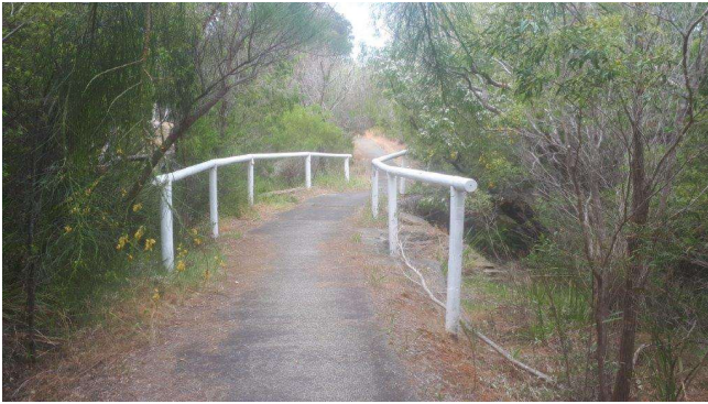
Figure 10. Photographs of existing culvert within application area (Shire of Augusta Margaret River, 2021).
