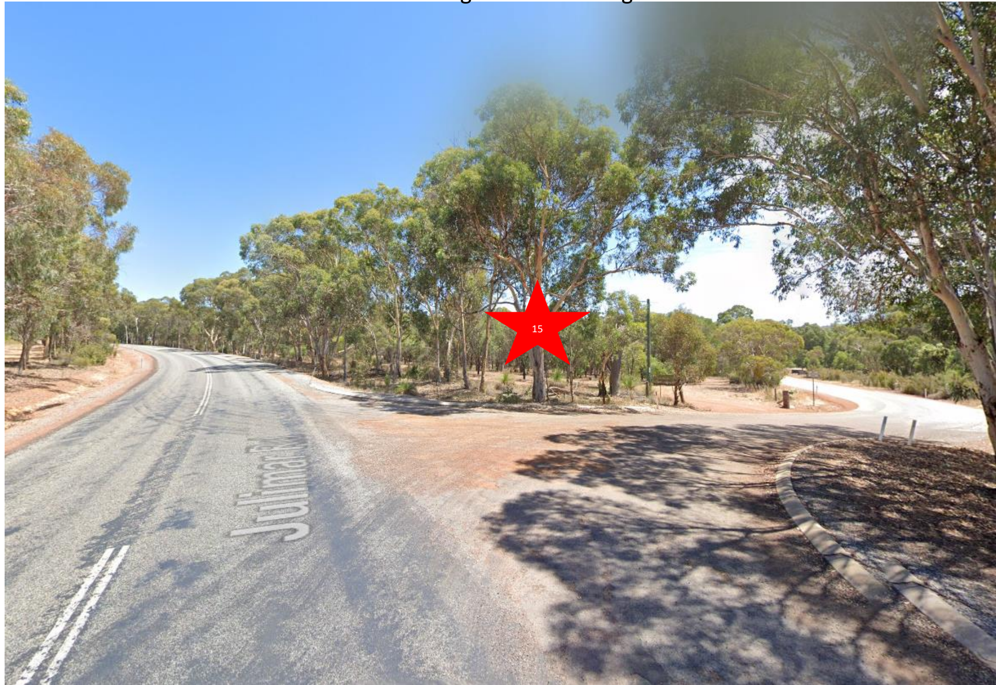
Tress obstructing culvert crossing headwall
