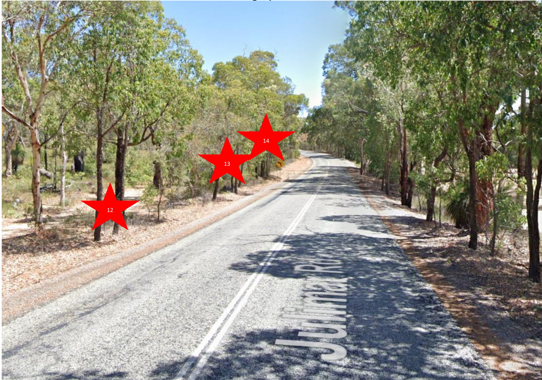
Tress affecting open drain/water flow
