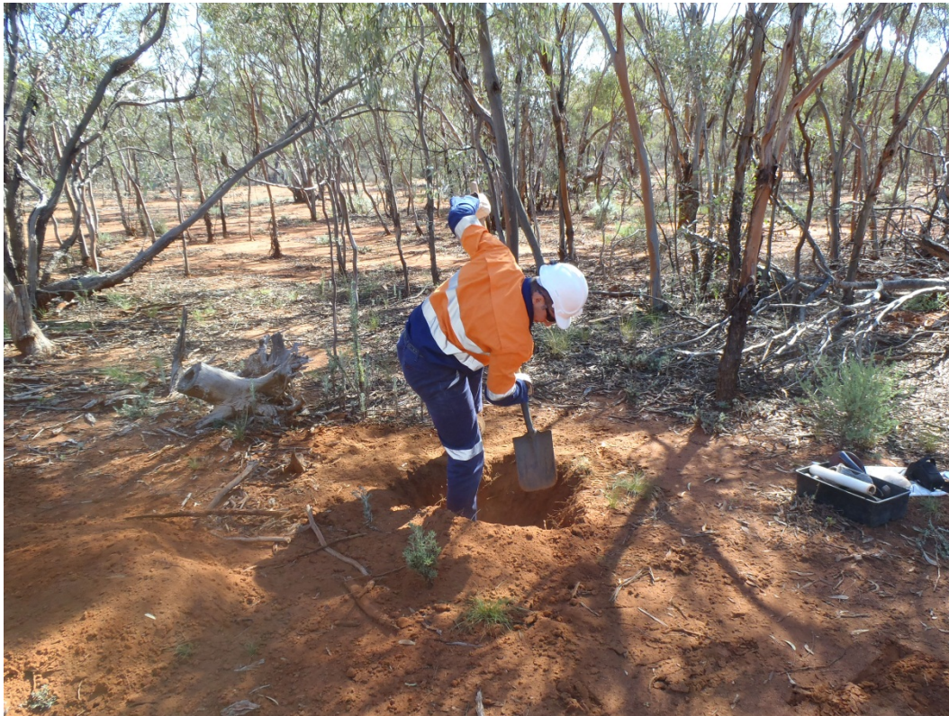
Plate 3.1: Excavation of shallow soil trenches by hand to characterise the surface soils.
