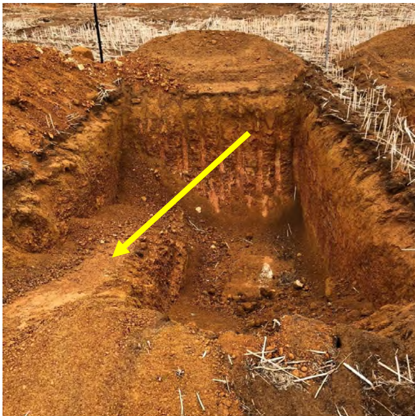
Figure 6: Example of egress ramp built on the left-hand side of the sump
