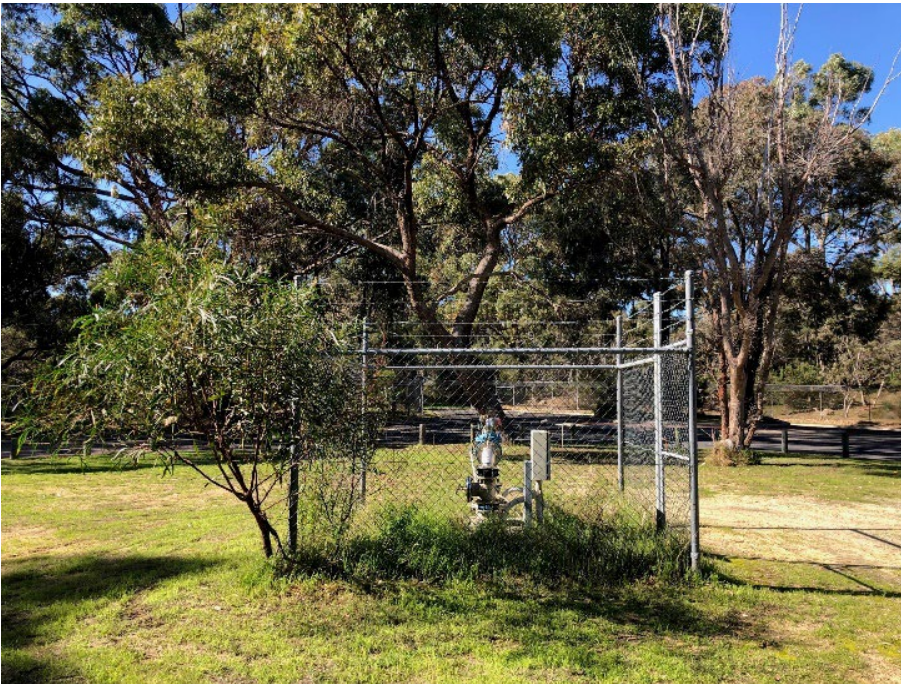
Plate 1: Geothermal groundwater bore (GWL 182271). The bore is, outside of clearing permit area however is included as it shows the commencement location for the pipeline.
