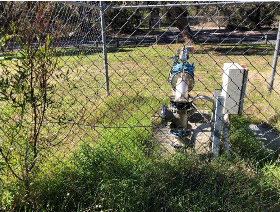
Plate 2: Close-up photo of the geothermal groundwater bore (GWL 182271).
