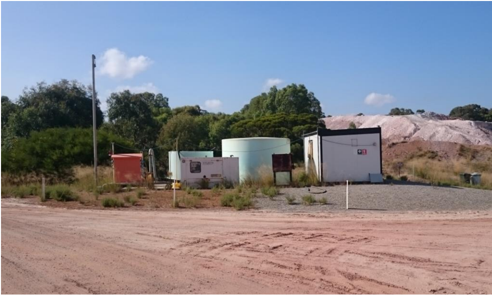
Pumping station for the vehicle washdown area and small lunchroom
