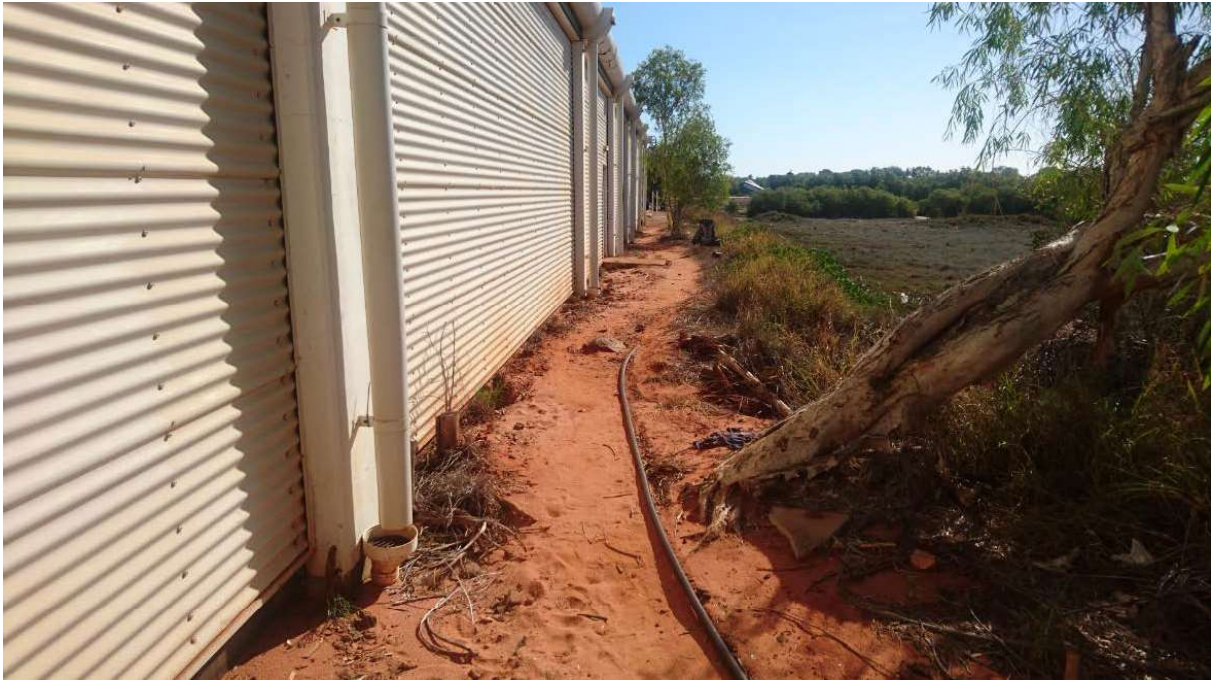
Figure 3.8: Rear of Paspaley Shopping Centre, showing reclaimed land level at foreshore edge of Dampier creek
