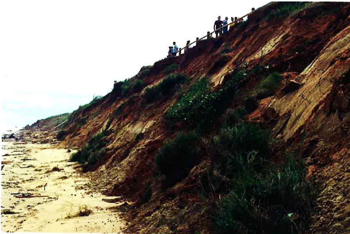
Figure 6.6: Post Cyclone Rosita – dune in front of Zanders café stripped back to Pindan Layer (Photo Shire of Broome)
