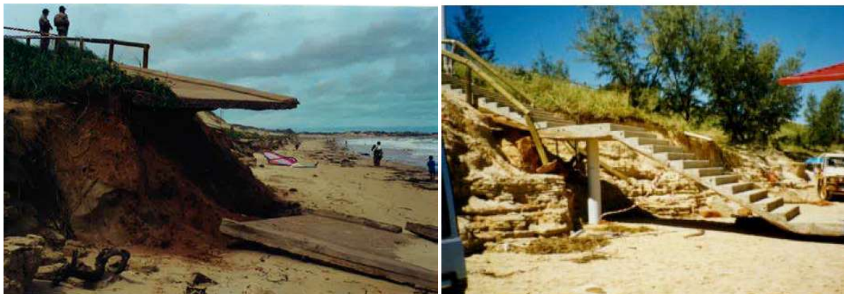
Figure 6.2: Cable Beach post TC Rosita 2000 showing (left) undermined beach access ramp and (right) beach access stairs (photo source: Shire of Broome, JCU 2000)
