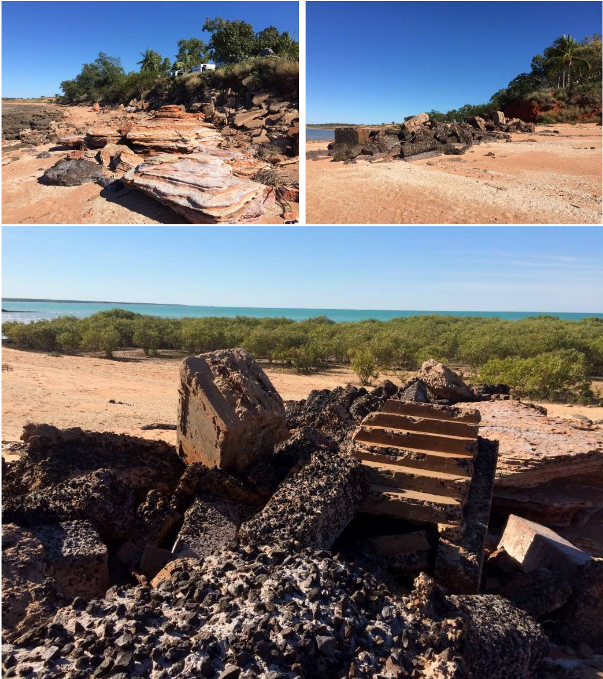
Figure 3.4: Shoreline protection in front of Roebuck Bay Caravan Park, Town Beach. Upper left Mix of native and placed rock in the foreshore at base of cliff, Upper right and lower: groyne structure at midpoint of caravan park frontage made of old building material.
