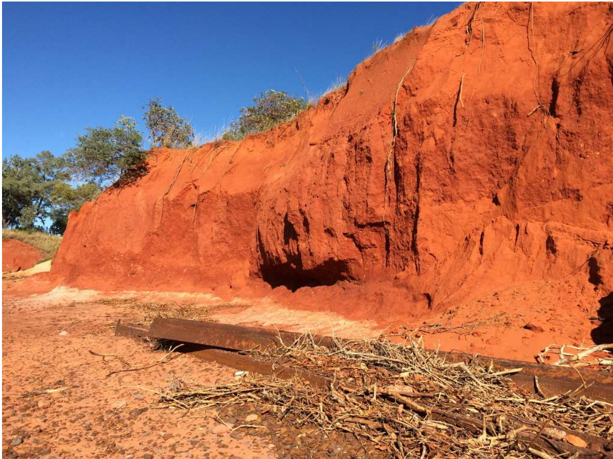
Figure 6.8: Town Beach eroding pindan cliff with example of undercut cliff base
