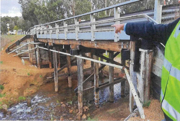
Photo 3: Services on LHS of Bridge 0256A
