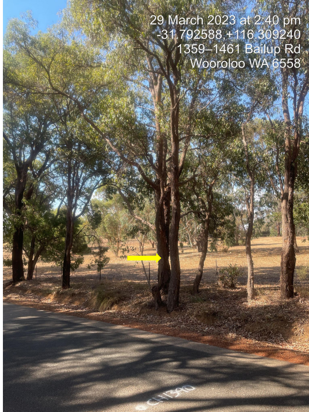
Remove – Tree in drain 300dia SLK 1.395 RHS *Tree can be retained if deemed significant or trigger for permit
