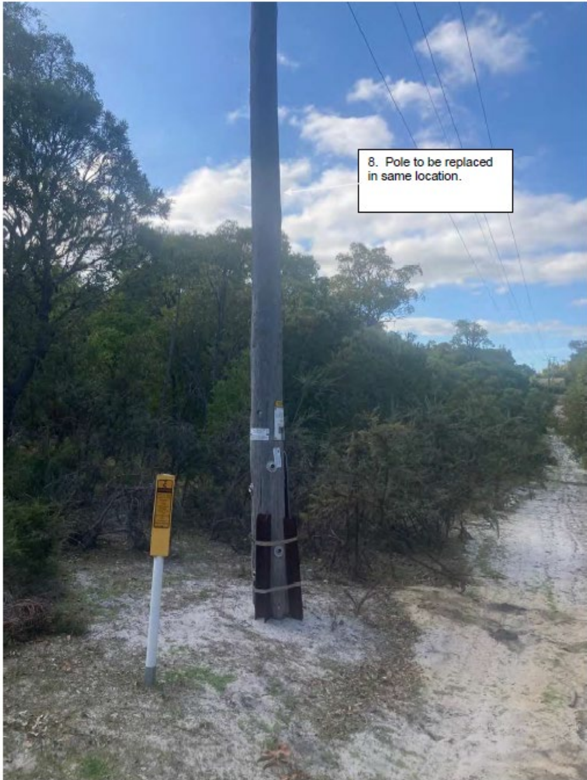
Figure 3: Pole S740404 to be replaced in its current location (10 m from I) in Construction Detail B (I to J)
