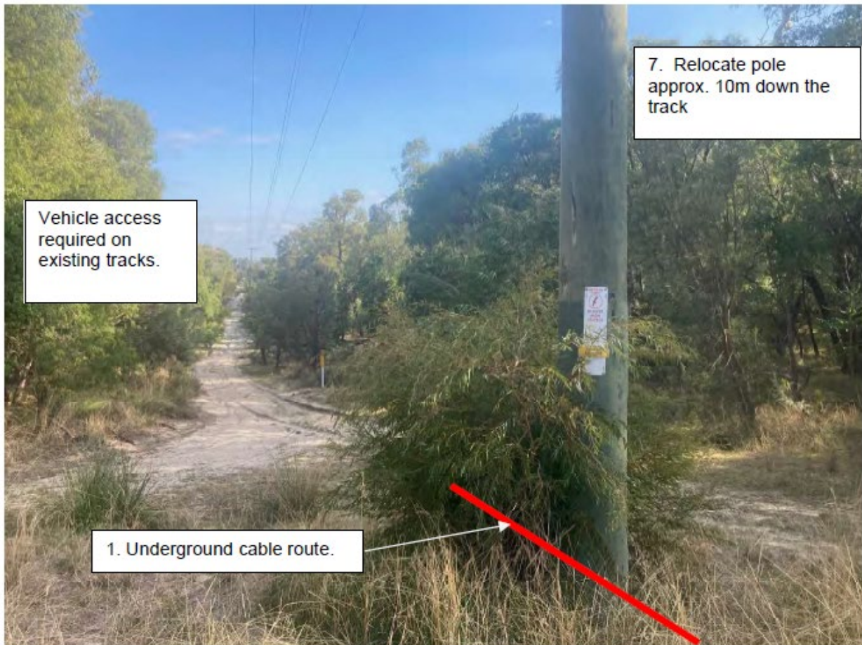
Figure 2: Relocation of pole S740403 (currently 10m from J) in Construction Detail B (J to I)
