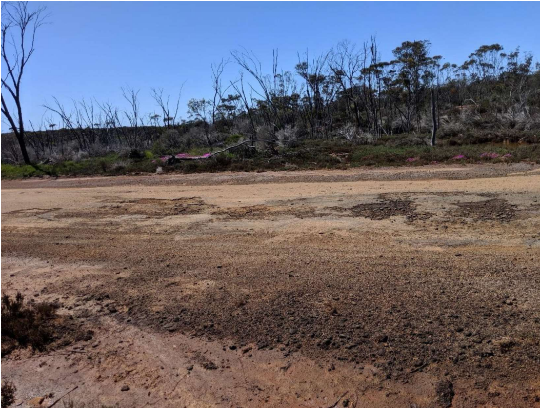
Figure 3. Photo showing poor condition of the Oldfield Road floodway. Photo taken by Katherine Walkerden on the 28/9/2022.
