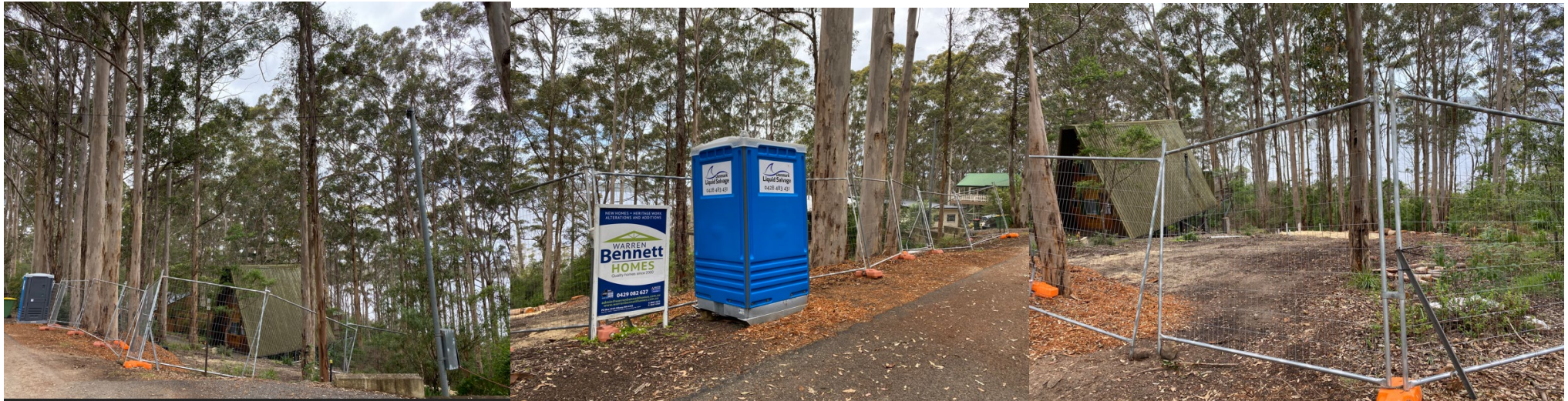
23 Payne Rd (A 711) – road verge and block understorey already completely cleared, road verge mulched.
