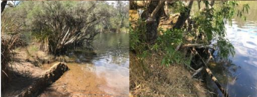
Boat ramp including a) relatively narrow (~3.5m) wide insitu concrete boat ramp and low cemented stone retaining walls of variable alignment, b) overhanging tree downstream and c) undercut bank near large tree upstream.
