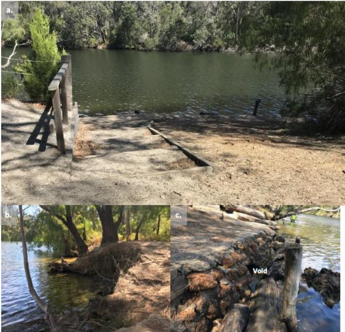
River Access 1 including a) compacted gravel stairs with timber supports and relatively steep sloped gravel bank, b) vertical undercut banks upstream which are sites of temporary boat mooring, and c) degraded cemented stone retaining wall with timber logs. Large void in wall in one area.
