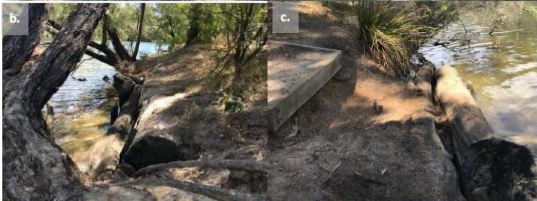
River Access 2 including a) compacted gravel stairs with timber supports b) stabilised bank to the north using timber logs, sloped upper embankment and fencing for managing pedestrian access, and c) undercutting of stairs and bank erosion.
