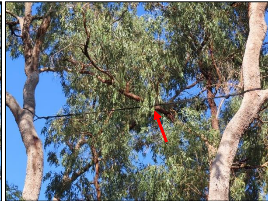
Image taken April 2024 Note the cable now looks slightly tauter compared to the Last Inspection
