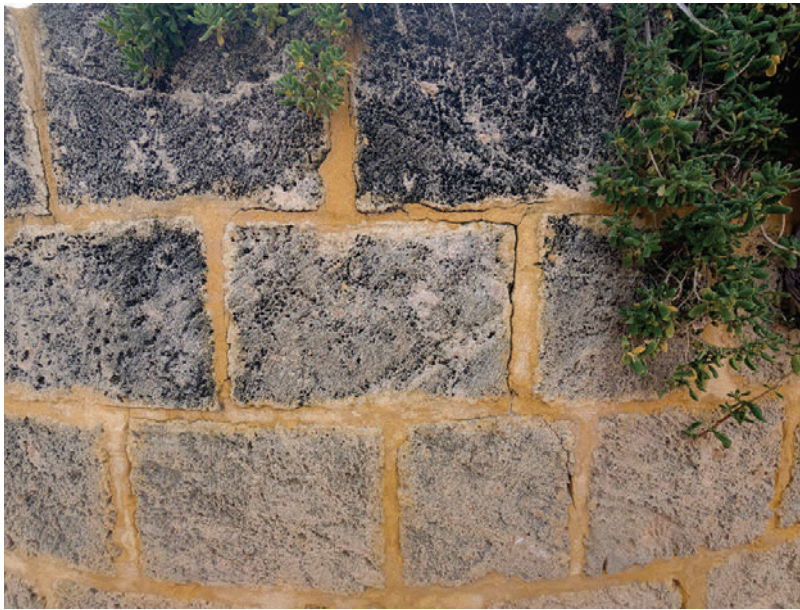
Plate 15: Example 2 of deterioration on limestone wall.
