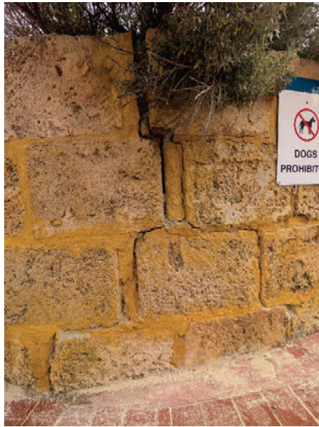
Plate 17: Example 4 of deterioration on limestone wall.
