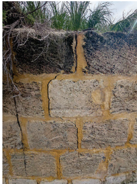
Plate 14: Example 1 of deterioration on limestone wall.
