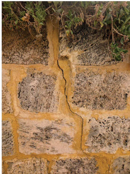
Plate 18: Example 5 of deterioration on limestone wall.
