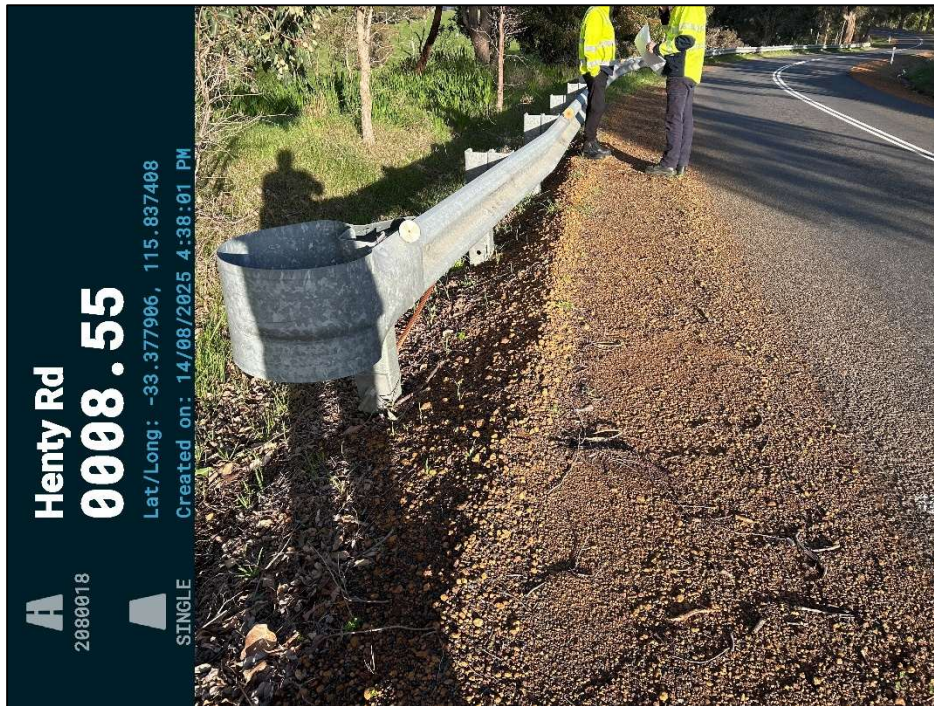
Finding 2.2 – The existing W Beam road safety barrier is not compliant to current standards (particularly the end treatments), however with new delineation provides a suitable treatment. If the barrier was damaged, then a new barrier to the current standard should be installed.
