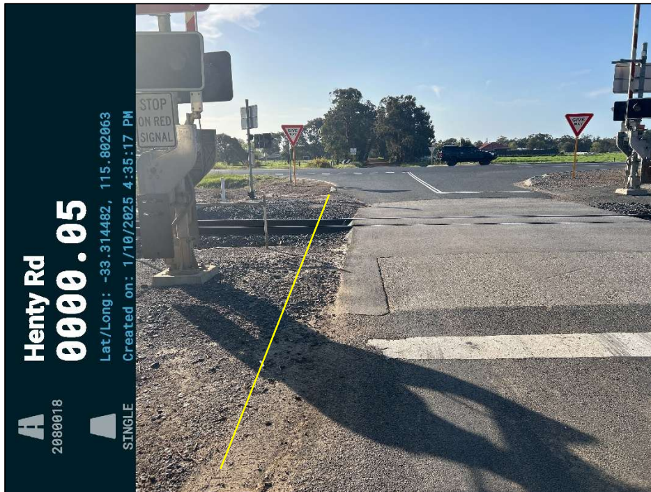
Finding 2.4 – The railway crossing is narrower than the sealed road pavement. Drivers may not realise the narrow section and drive over the rails.
