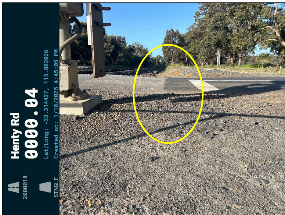
Finding 2.4 – The railway crossing has a dip where the culvert is located, this should be made smooth.
