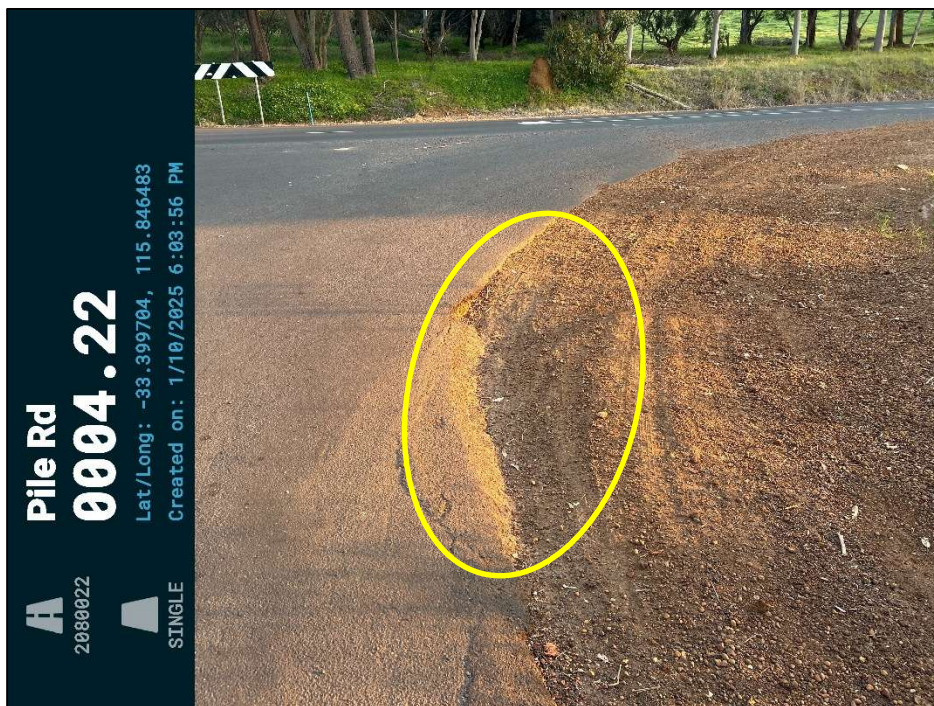
Finding 2.9 – A section of the existing shoulder has deteriorated due to vehicles cutting the corner. The swept path for the design vehicle should be confirmed and widened if required. If vehicles are using the gravel shoulder to travel faster through the curve, then kerbing should be considered to keep the vehicles on the correct alignment. Note, drivers may be travelling too fast from Pile Road into Henty Road due to other vehicles following them and the lack of a deacceleration lane on Pile Road.
