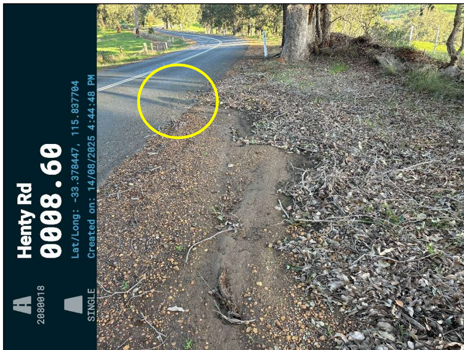
Finding 2.5 – The table drain is blocked, causing the water to flow over the road.
