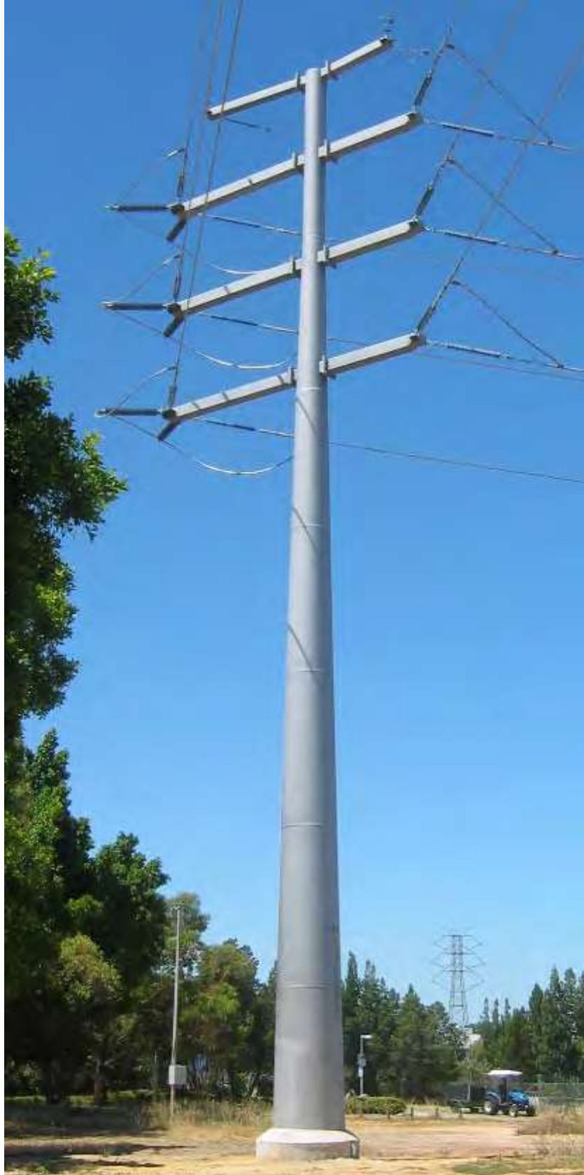
Figure 7: Double Circuit Steel pole
