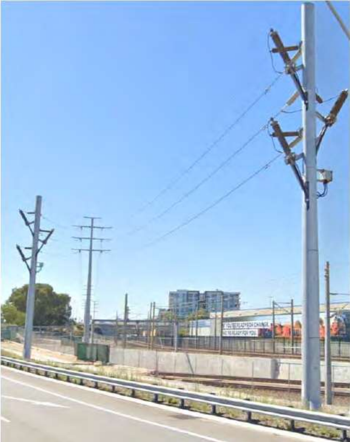
Figure 9: Double Circuit Steel pole with two transition poles
