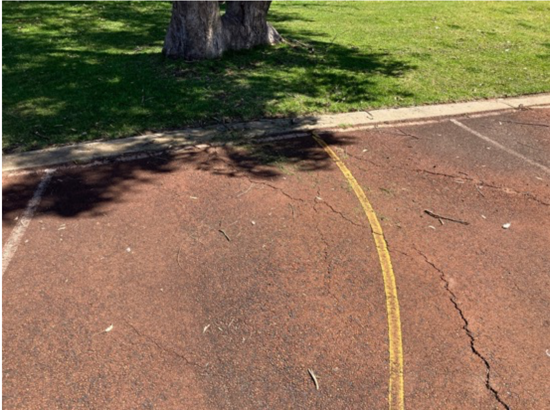
Figure 5: Mounding and cracking of the Basketball Court surface.
